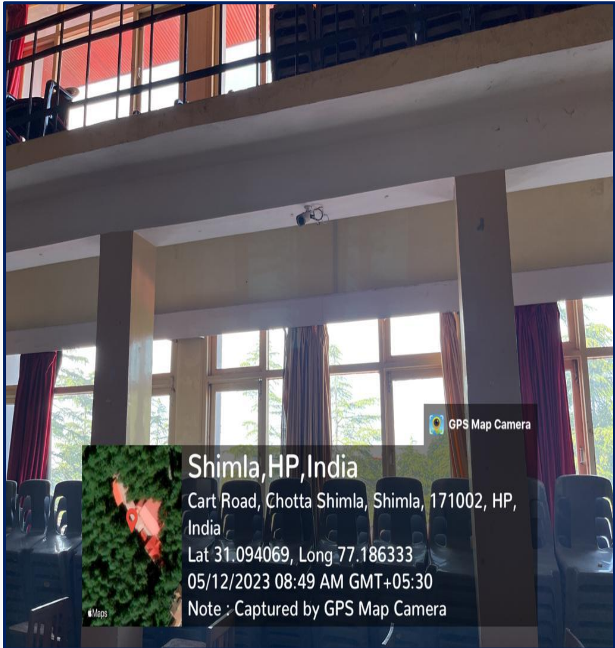
CCTV cameras installed throughout the campus
