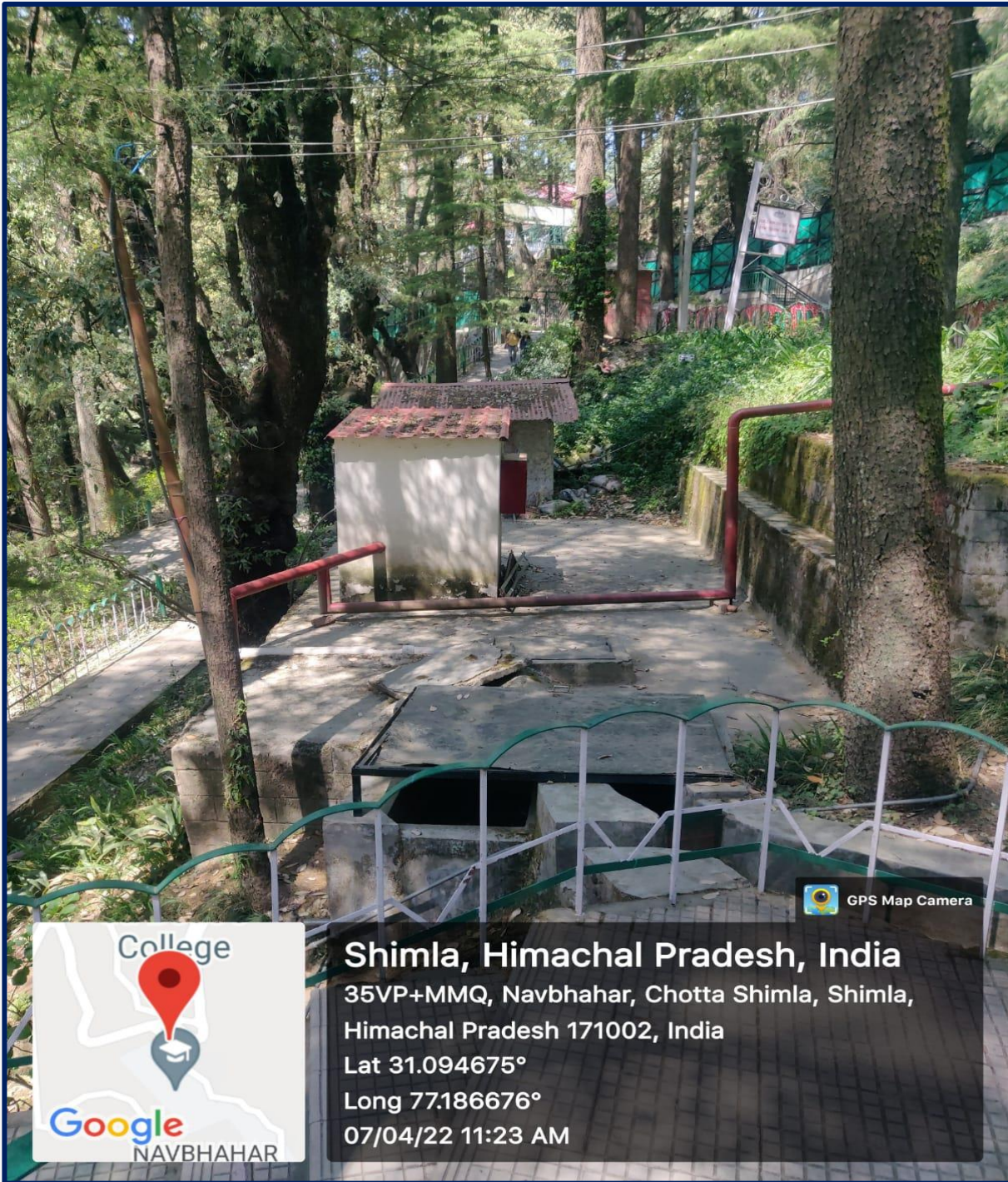
Rainwater Harvesting System
