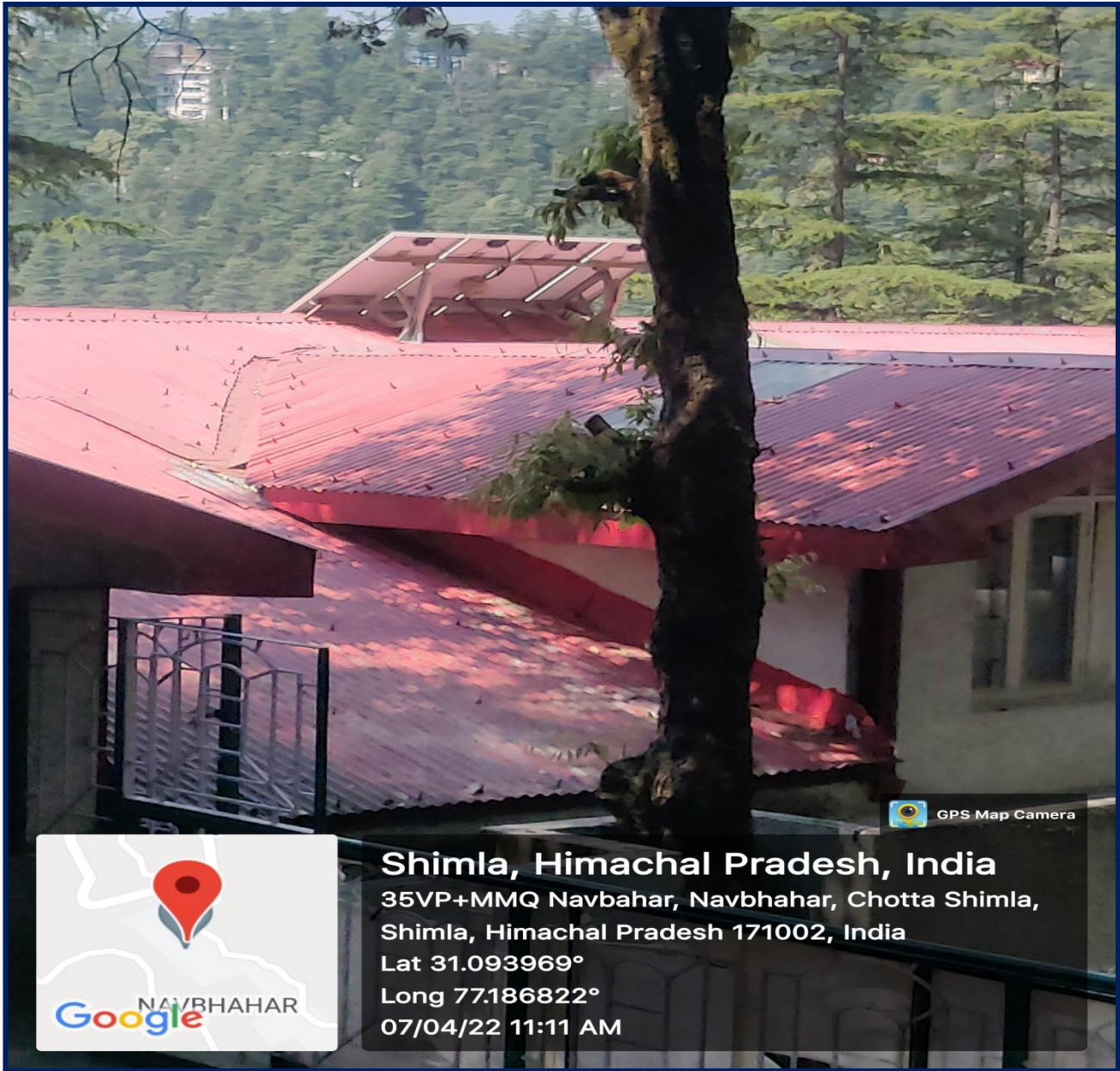
Solar Water Heater
