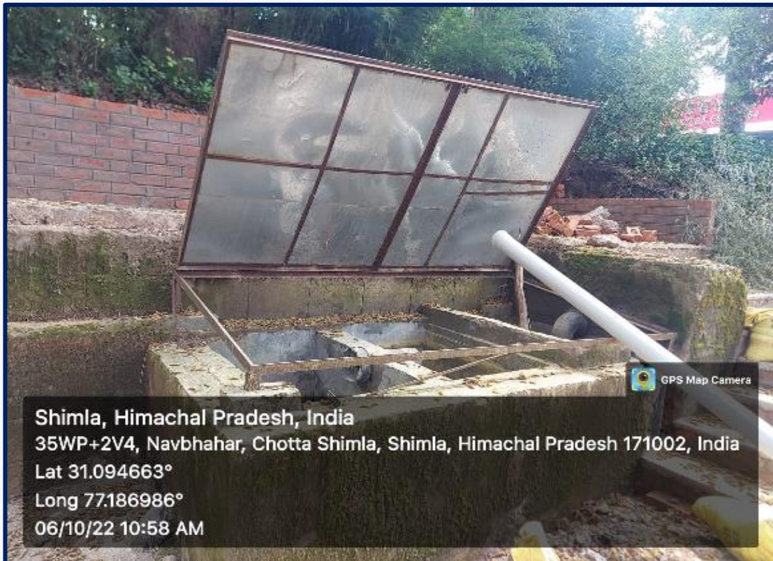
Rainwater Harvesting System
