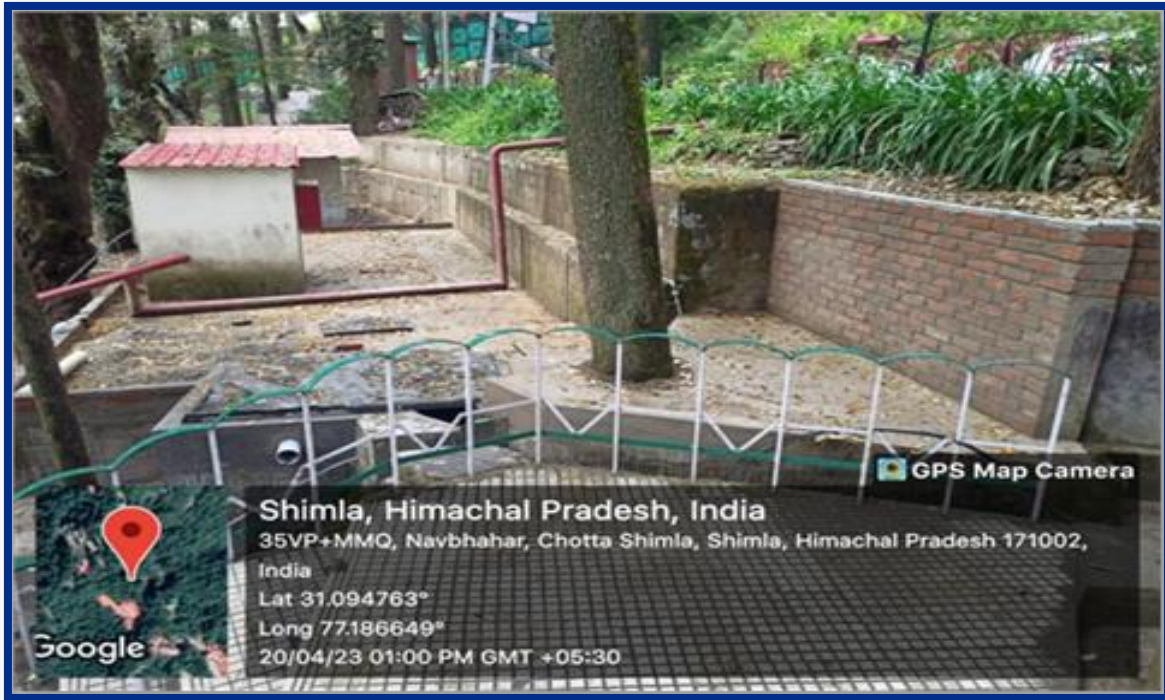
Renovated Rainwater Harvesting Unit
