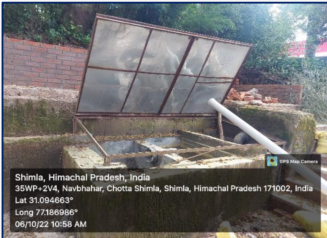
Rainwater Harvesting System
