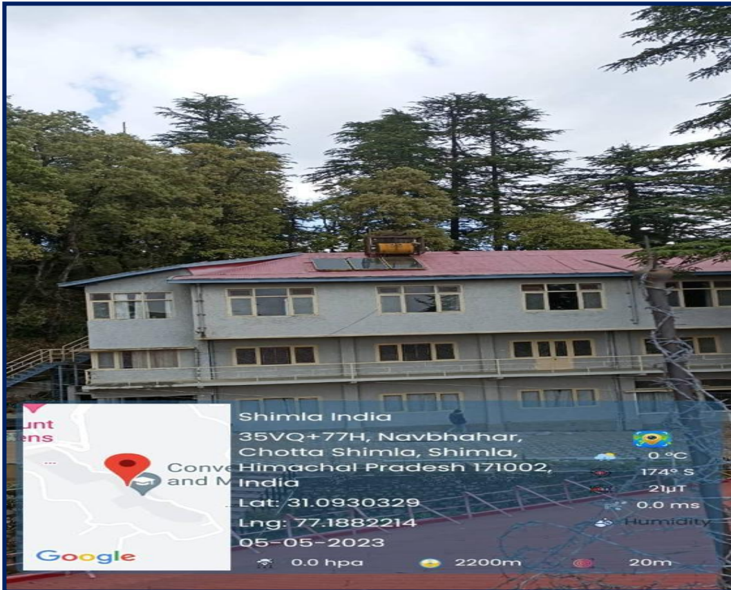
Solar Water Heater
