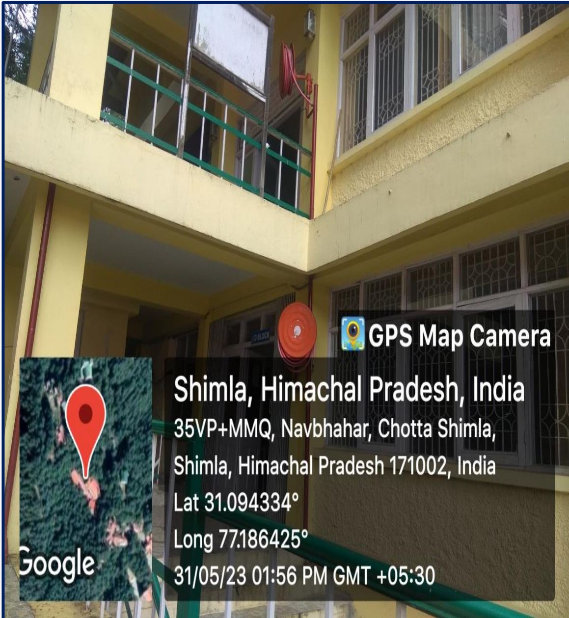
Fire Hague System
