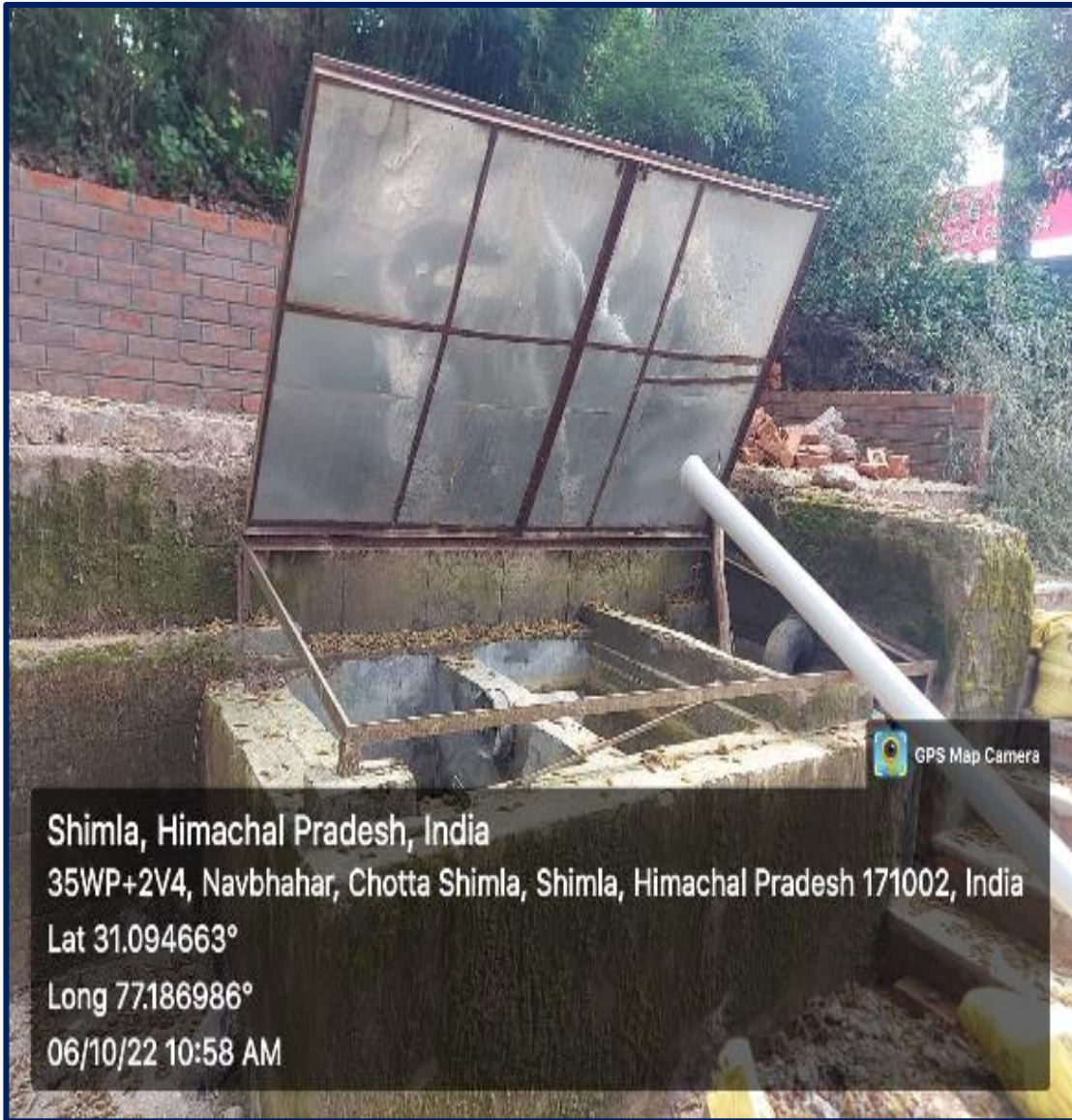
Rainwater Harvesting System
