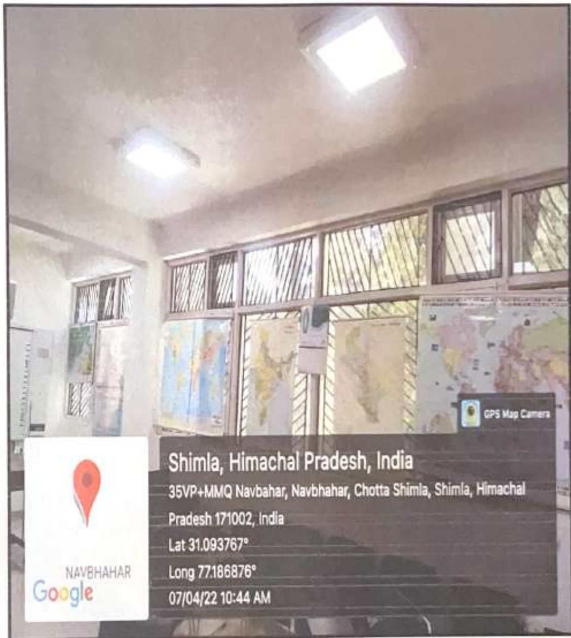
LED Lights in the Classroom
